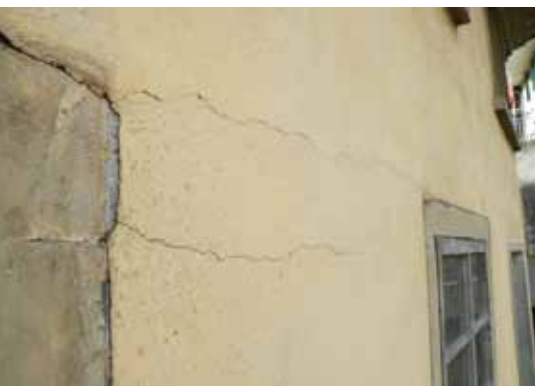
Fissures de joints
